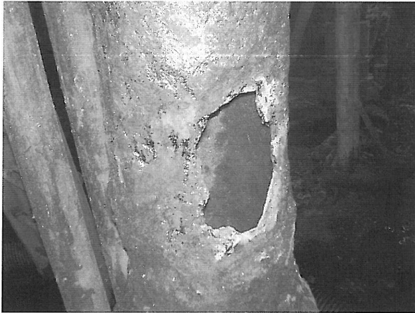
Hole in the discharge piping in Central Wet Well
