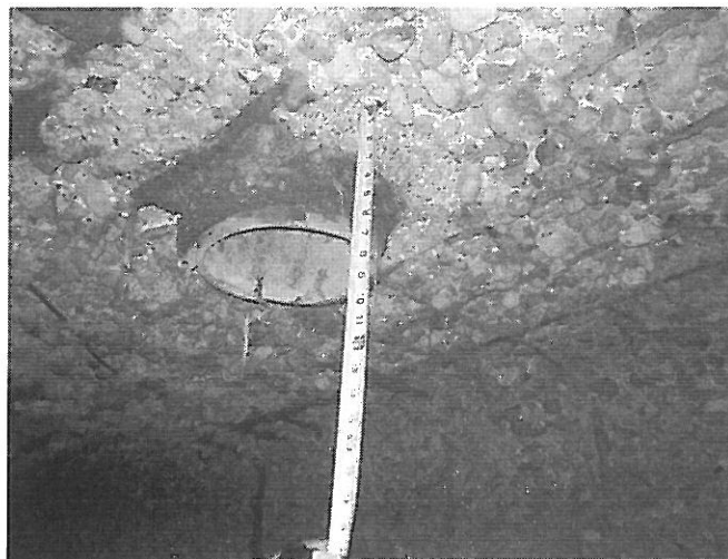
Approximately 5" of concrete surface removed from the Central Wet Well Ceiling
