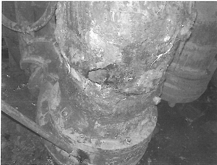
Corrosion on pump inside of Central Wet well
