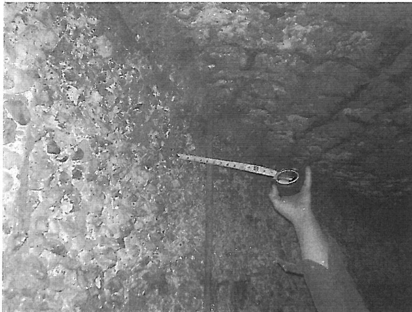
Approximately 5" of concrete corroded from Central Wet Well wall
