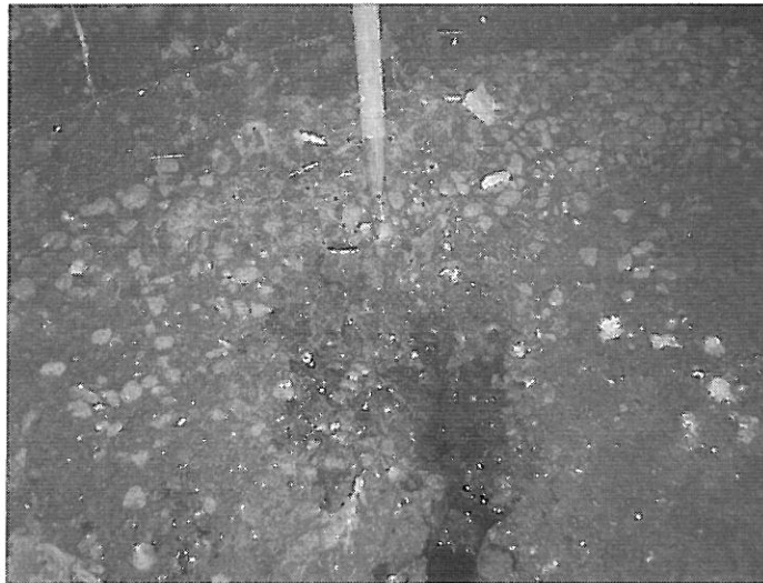
Approximately 6" to 7" of concrete aggregate on the Central Wet Well Floor
