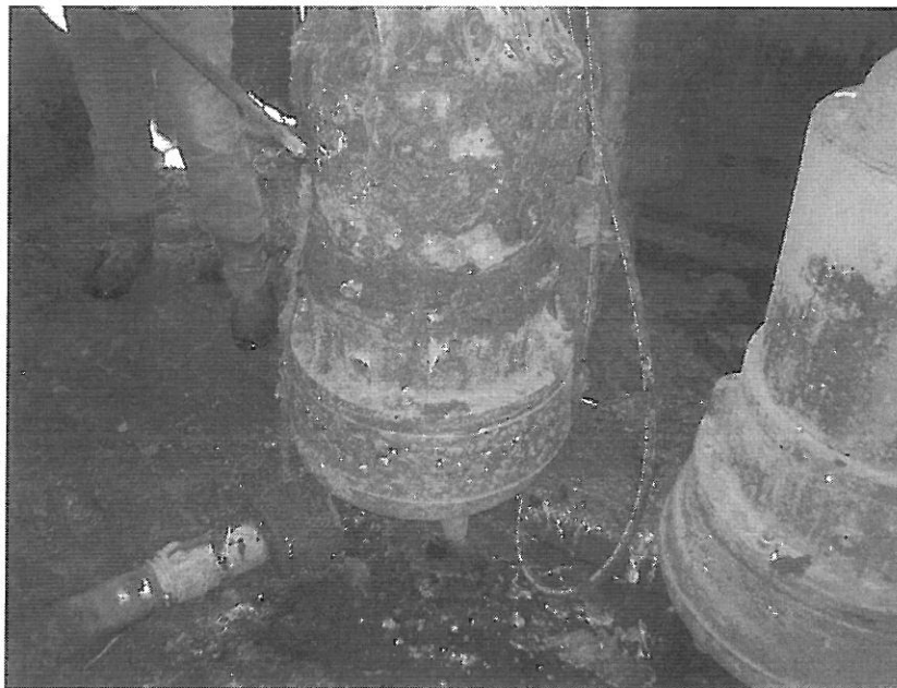
Hole in pump jacket in Central Wet Well
