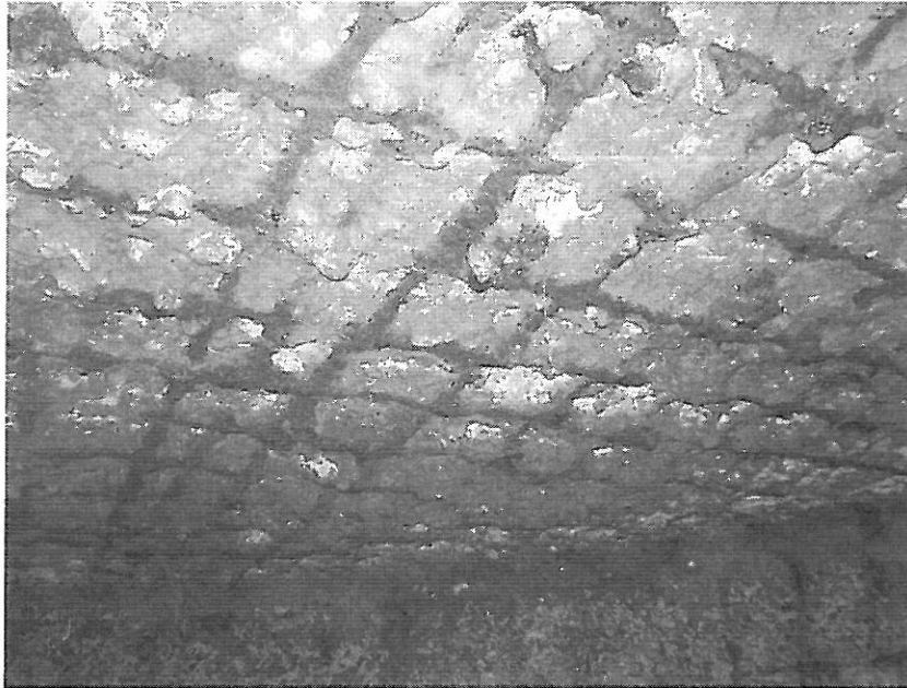
Reinforcing steel exposed in the Central Wet Well Ceiling
