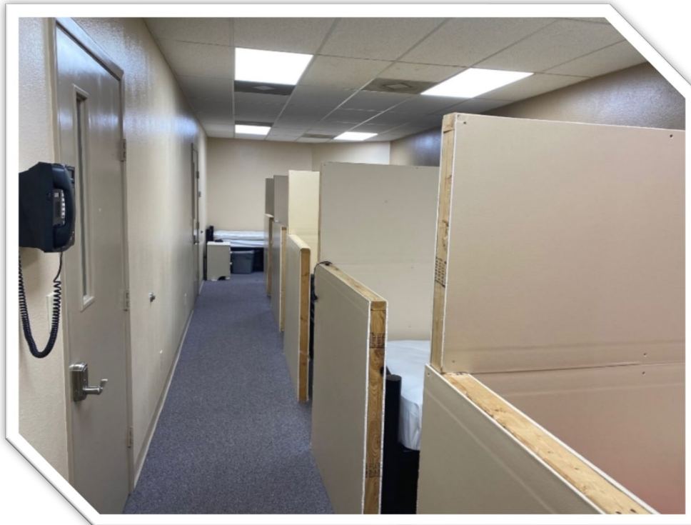
Barracks (sleeping quarters) need to be finished at Station 1
