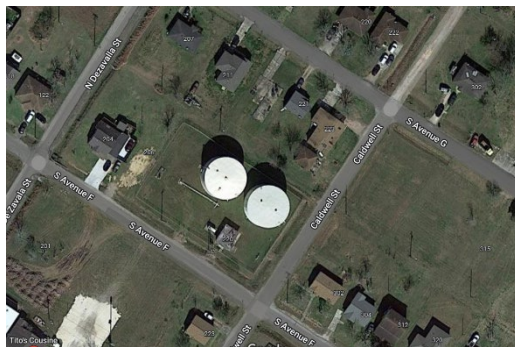
F Avenue Booster Pump Station
