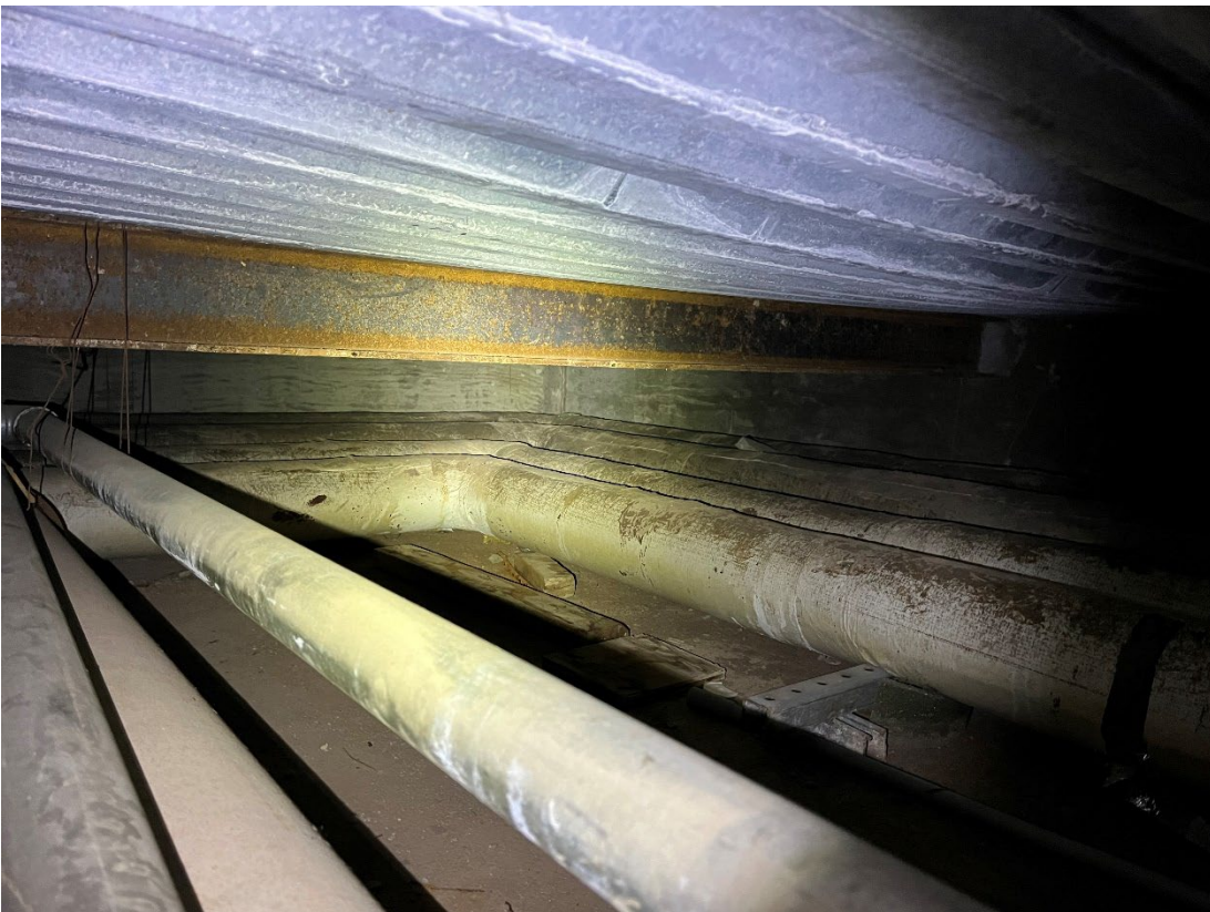
Photo #4: View of pipe fittings inside the vault area
