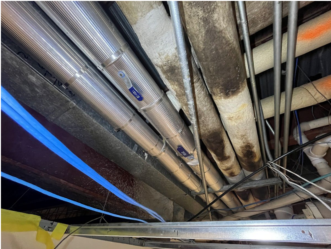
Photo #22: View of piping on Level 2 – lobby area near vertical pipe chase.
