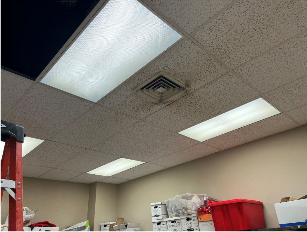
Photo #21: View from beneath asbestos ceiling tiles in Vault D.
