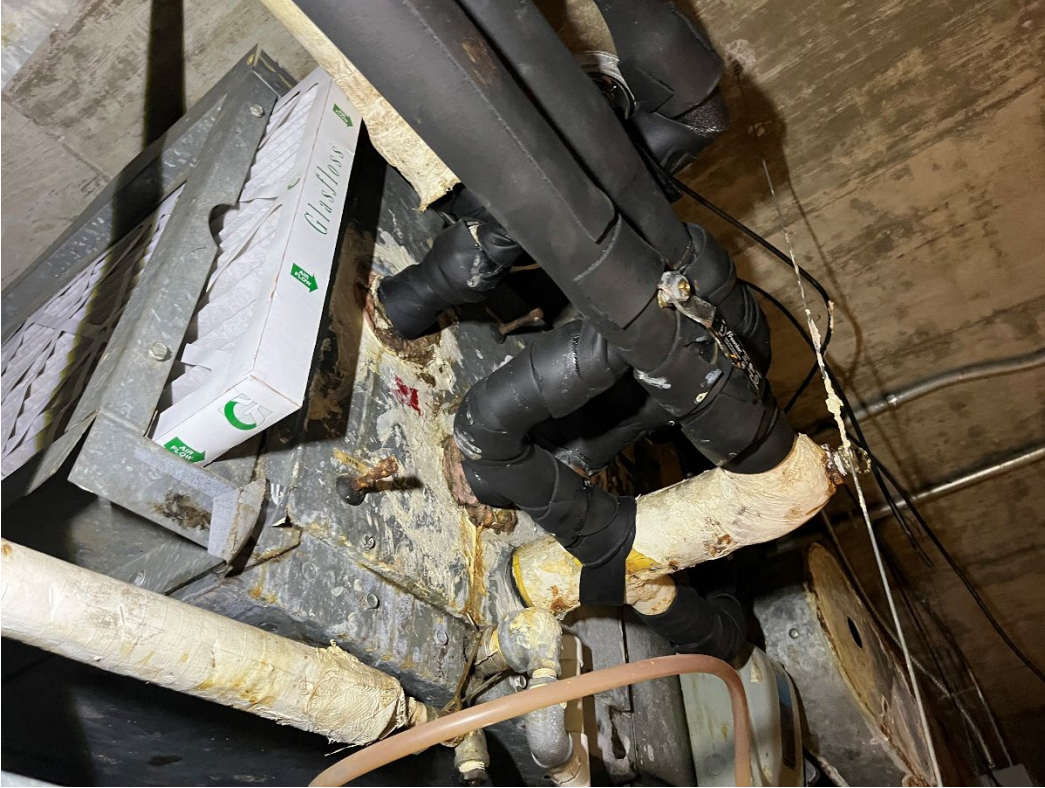
Photo #17: View of air handler unit and piping – Level 1 – Vault D.
