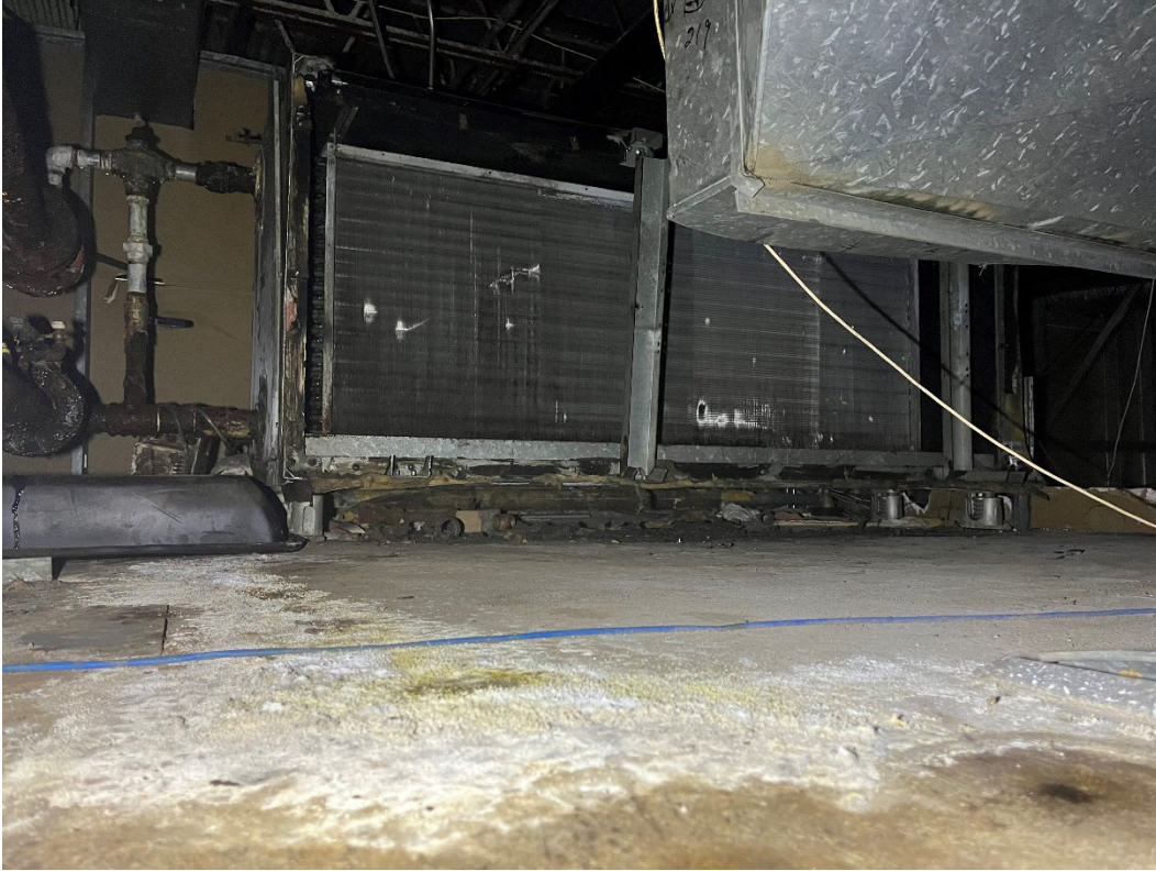
Photo #27: View of evaporator coil and framing – above Vault 1.
