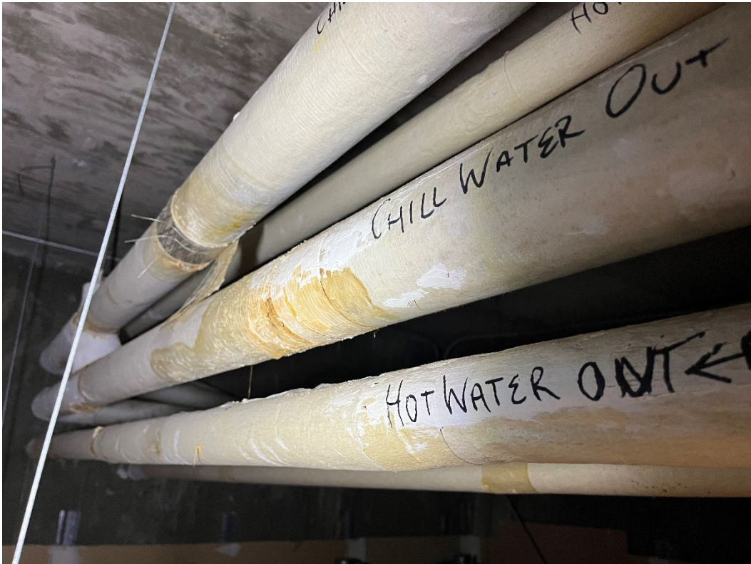
Photo #16: View of piping runs in Level 1 – Vault D.
