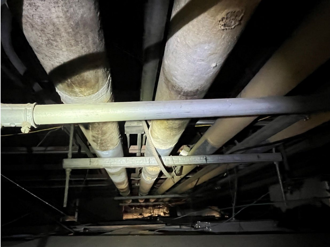
Photo #9: View of the piping runs, above Level 1 lobby areas, rooms 116-117.
