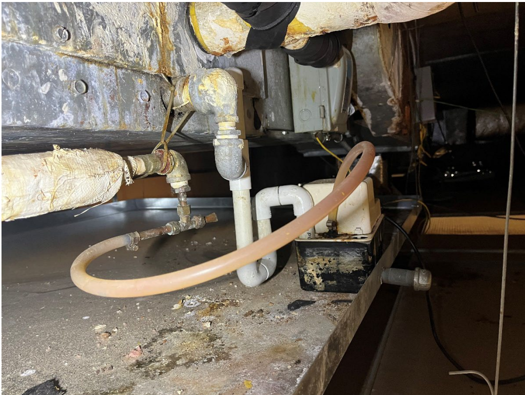
Photo #18: View of air handler and piping – Level 1 – Vault D.
