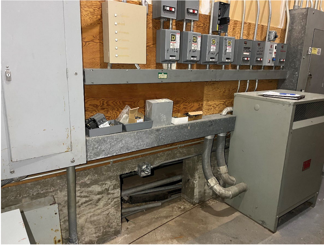
Photo #1: Level 1 – Mechanical Room – Behind Elevators
