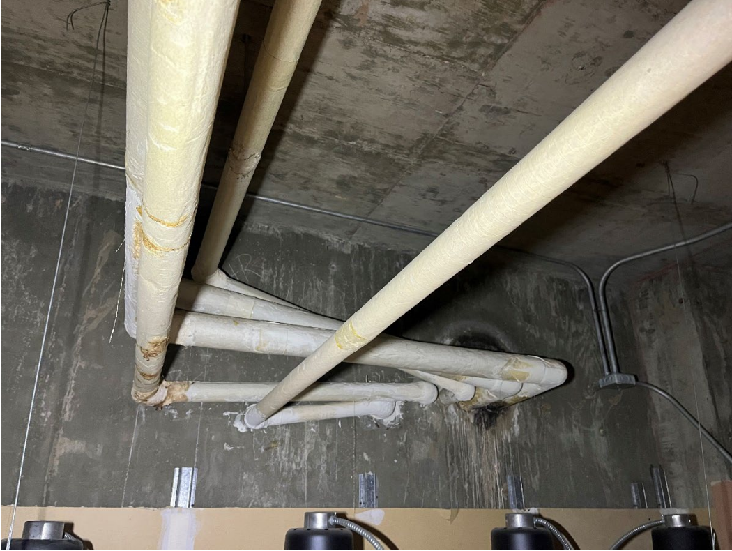
Photo #15: View of pipe fittings in Vault D – Level 1.
