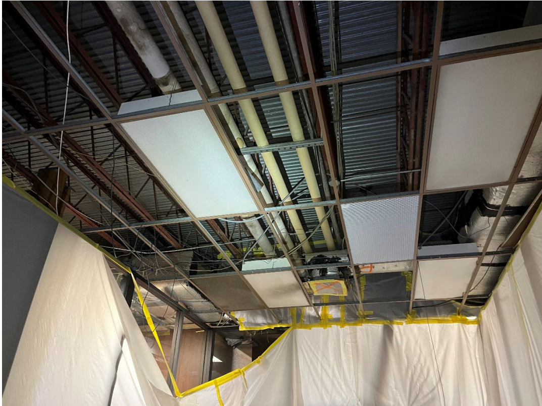
Photo #11: View of the piping runs – Level 1 – Room 126.
