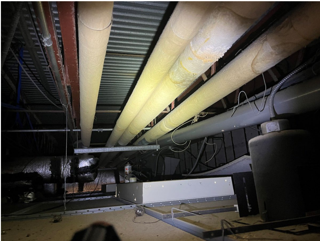
Photo #14: View of piping runs above tellers and room 115.
