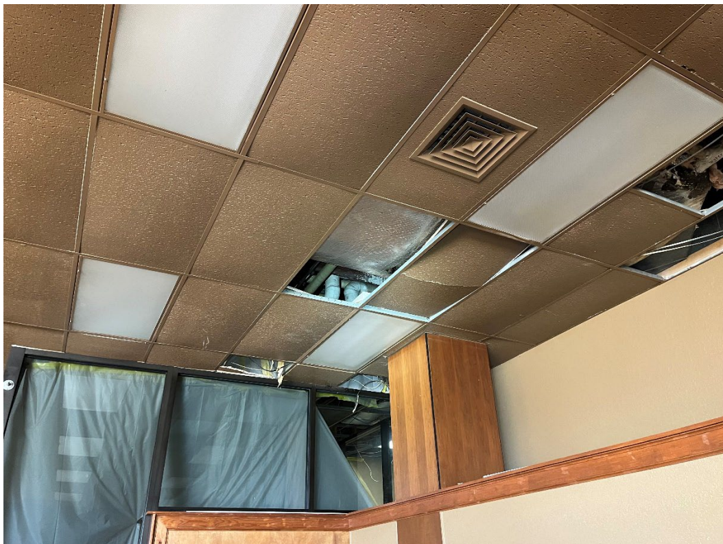
Photo #12: View of pipe fittings above ceilings – Level 1 near room 131.
