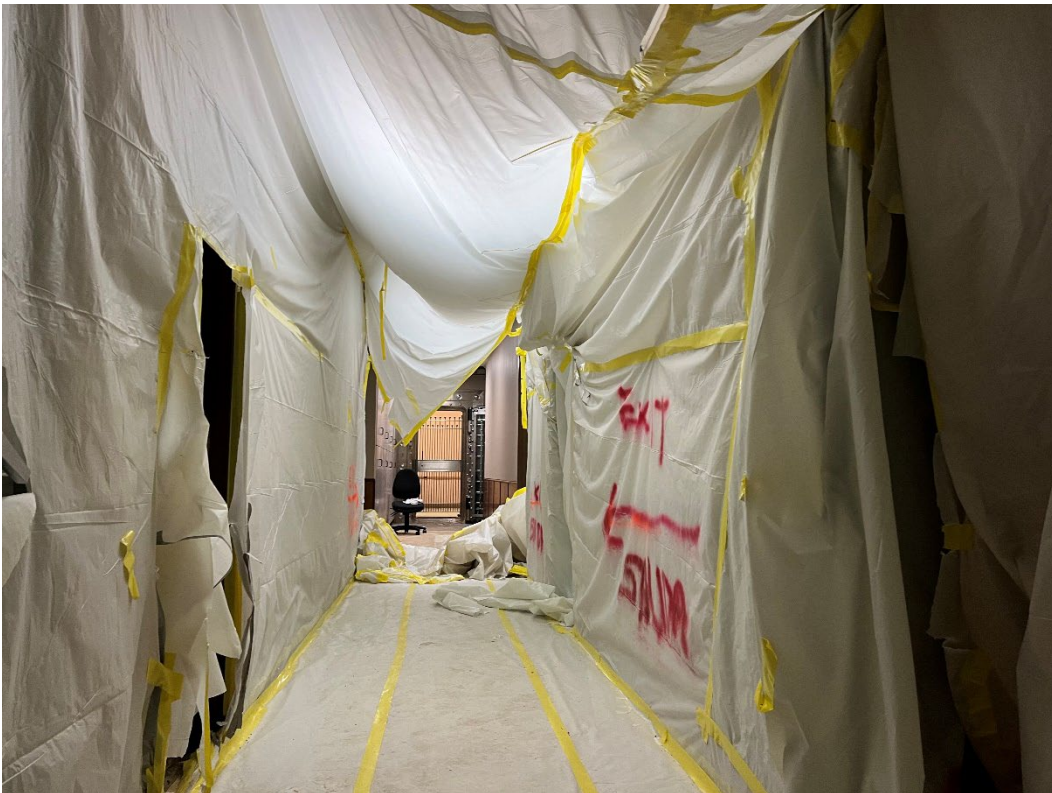
Photo #30: View of remaining poly from previous abatement contractor.
