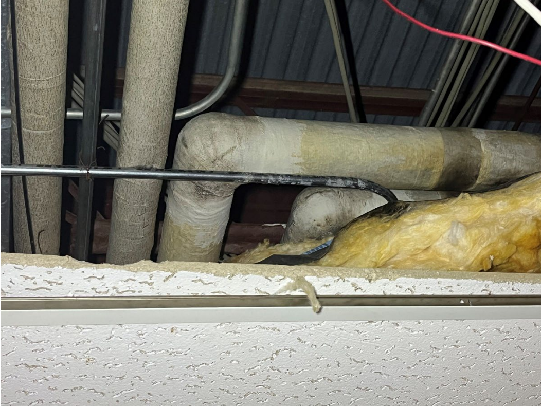
Photo #25: View of piping above utility closet.
