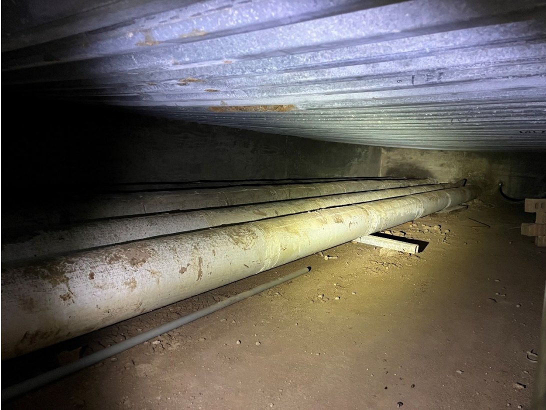
Photo #3: View of piping entering the vault – northwest vault area.
