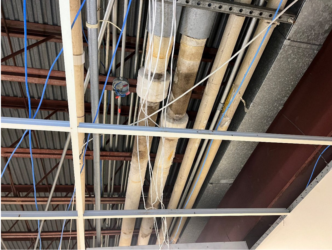
Photo #23: View of pipe fittings in Level 2 lobby area.
