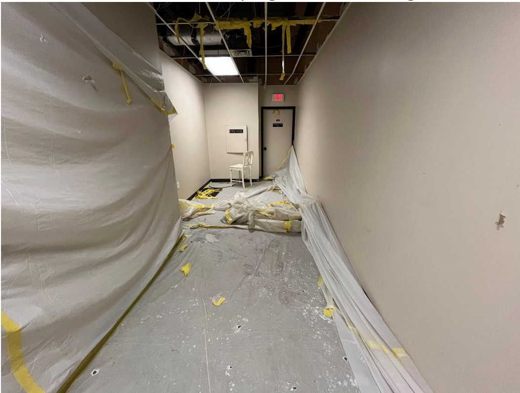
Photo #29: View of remaining poly from previous abatement contractor.
