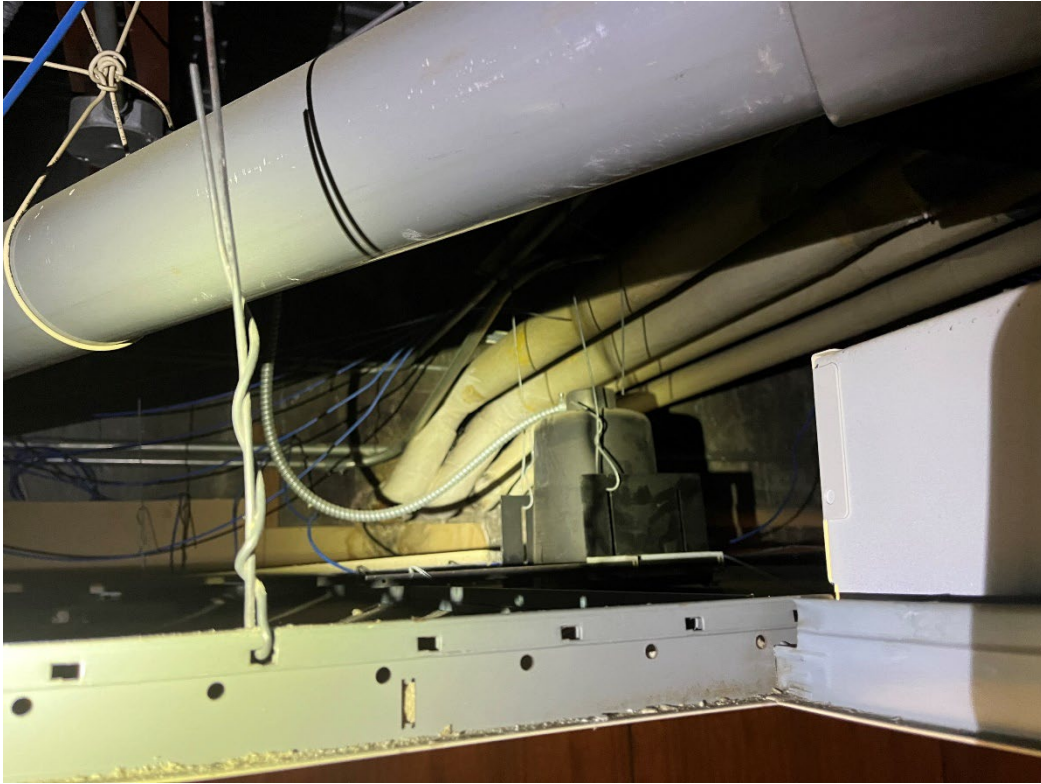
Photo #13: View of pipe fitting near wall penetration, south wall of room 113.
