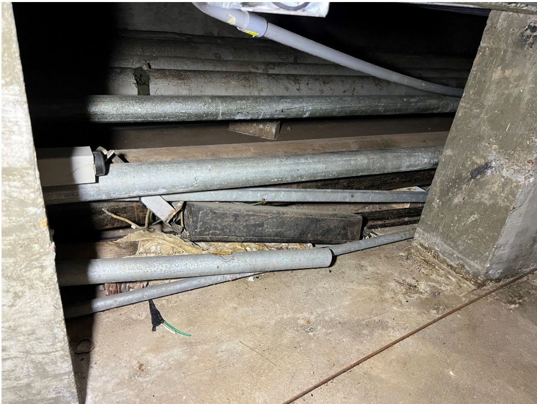
Photo #2: View of Piping Vault Access in Mechanical Room
