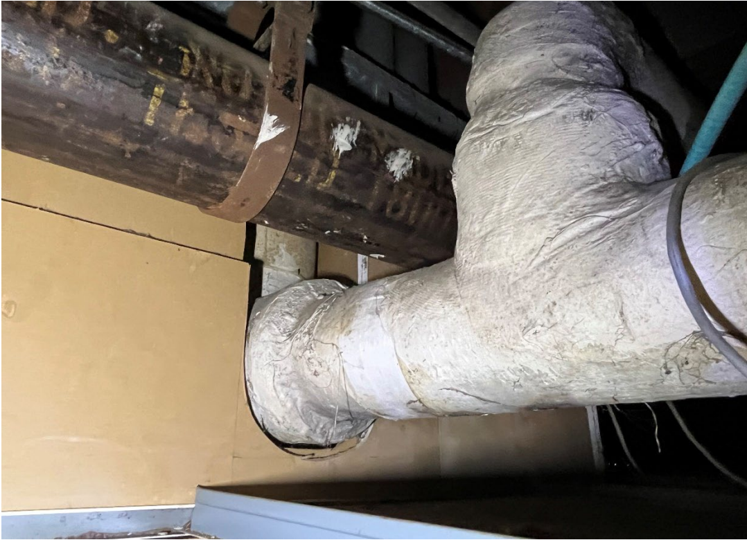
Photo #7: View of pipe fittings above Level 1 ceiling.
